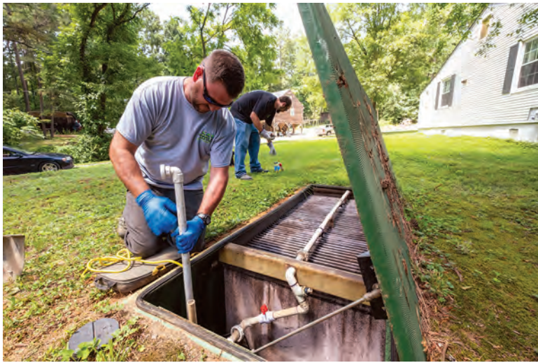
Billy Shaw, foreground, and Ed Schneck provide maintenance to an AdvanTex system from Orenco Systems.
