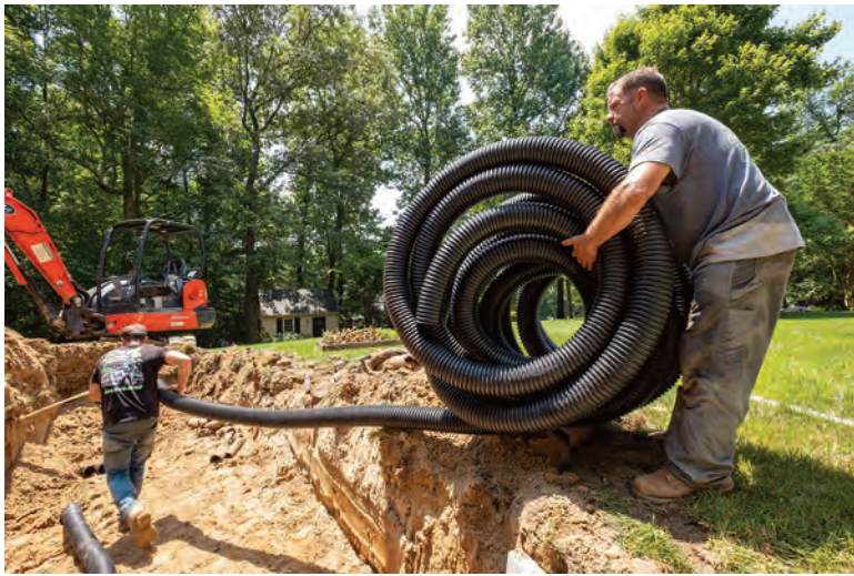
Jimmy Butler, left, and Shawn Riggs lay out new corrugated plastic lines to replace those clogged with sediment.
